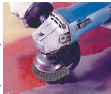
Removing paint from a steel surface with a crimped wire cup brush.
